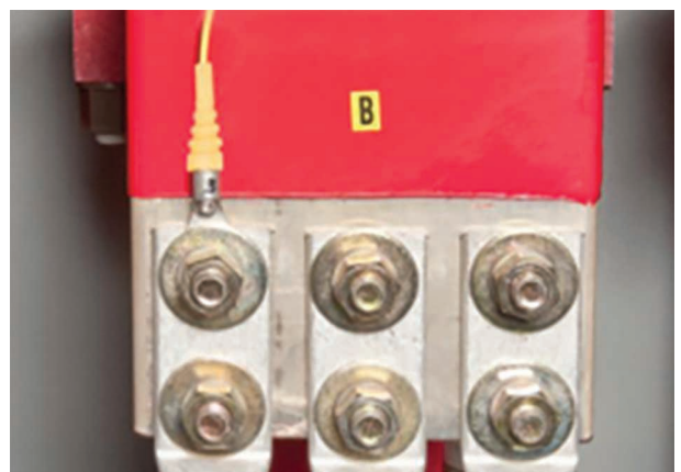
FIGURE 7. A fiber-optic sensor secured under a bolted electrical connection.
