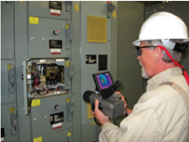
FIGURE 1. A thermographer conducting an IR Scan of a low-voltage MCC unit. Note the door interlock has been defeated to allow the equipment to remain energized with the door open. (This image predates protective clothing requirements for energized work.)
