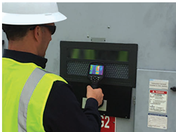
FIGURE 5. IR windows are available in various sizes and geometries to capture a broader view for thermographic images without exposing personnel to energized equipment.
