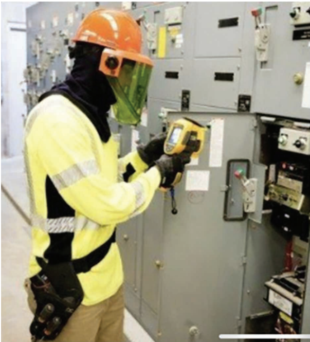
FIGURE 2. A hand-held IR device inspecting electrically energized equipment to allow meaningful operating data to be captured.
