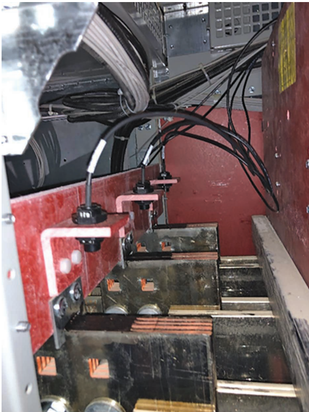
FIGURE 8. Noncontact IR sensors targeting bus connections for continuous thermal monitoring.
